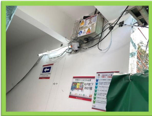
Motion sensors for lighting system
